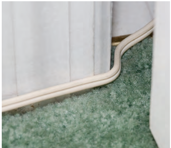
Damaged/bent cords can cause arcs
