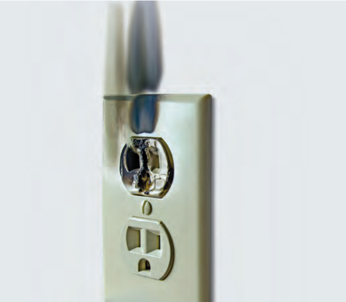
50 to 75 percent of all electrical fires in the United States are caused by arc fault conditions
