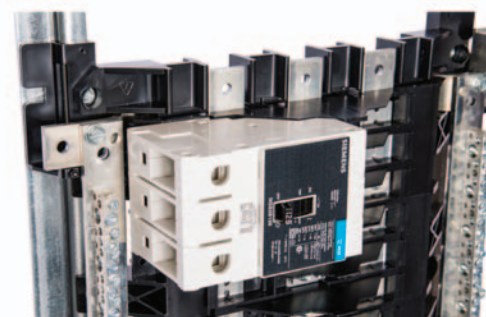
Example of Back-fed xGB Main breaker installed
