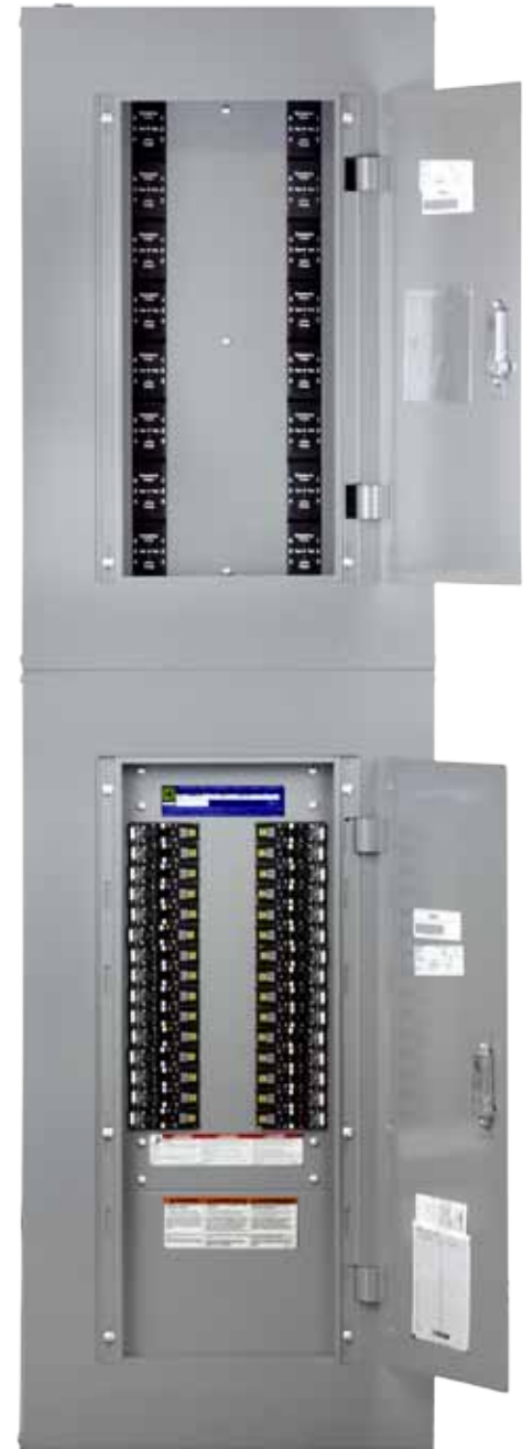
Emergency Lighting Control Panelboard
