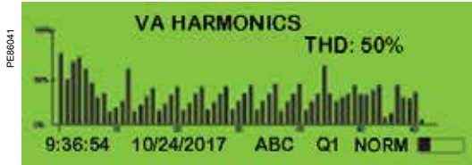
PowerLogic ION8650 front panel harmonic display.
