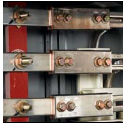
Horizontal Bus Splice
