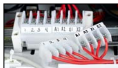
Control Terminal Block
