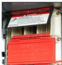
Automatic Vertical Bus Shutter
