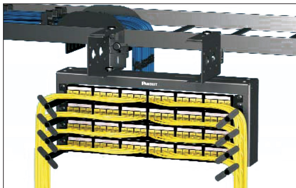
Mounted to side rail below ladder rack
