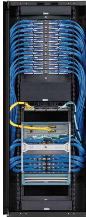
Converged Infrastructure for Nexus 7009 "Heavy Copper"
