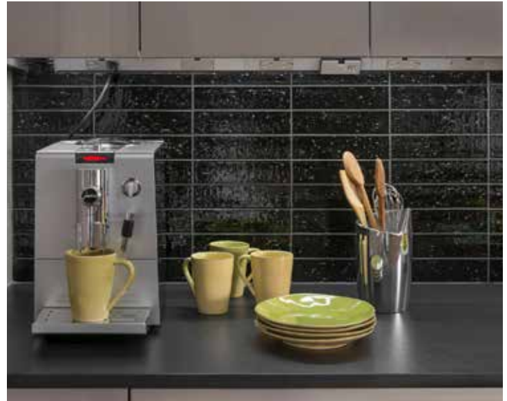
Under-Cabinet Lighting System installed in a kitchen.
