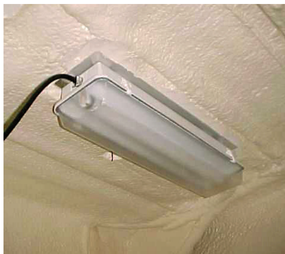
Single Light Package (Installed)
