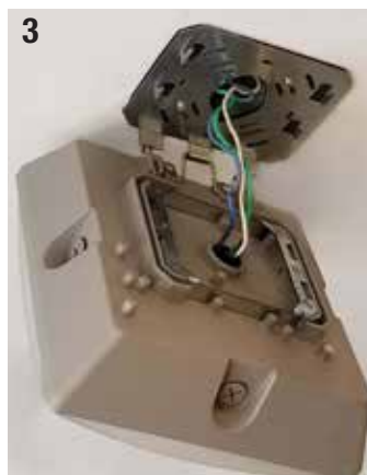
Complete wiring connections.
