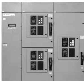
Next Generation AMPGARD Lineup— Front View
