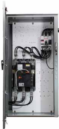
Enclosed S611 with Breaker Disconnect
