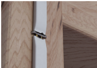
Tight staple can pierce insulation
