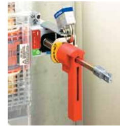
Door open: A strong metallic padlock kit allows up to three padlocks. The padlocking means is easily accessible, when locked closing of the disconnect is not possible.
