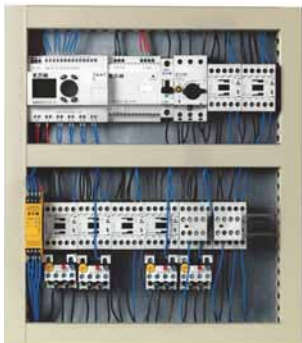
Panel with four traditional starters installed: FVNR, FVR, FVNR with E-stop and FVR with E-stop
