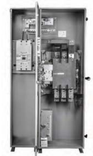
Separate Compartment for ATS and Breaker
