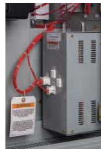
Multi-Tap Control Power Transformer
