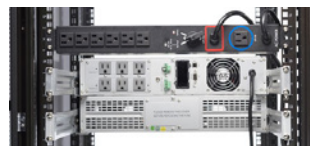
HotSwap MBPs rackmounted horizontally in rack
