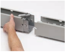
Install inside connector in wireway ends and tighten
